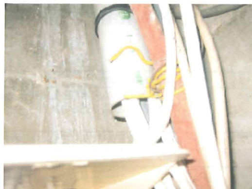
8310_GAINE TECHNIQUE Batiment B1
