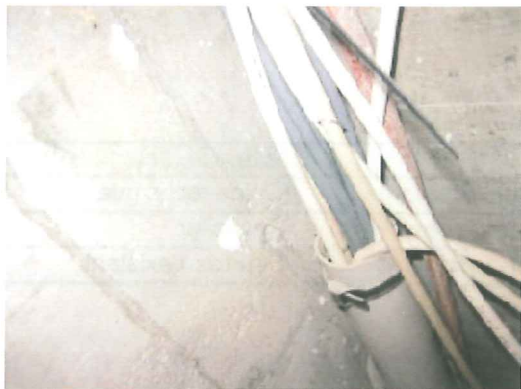
8309_GAINE TECHNIQUE Batiment B1
