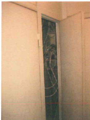
8295_GAINE TECHNIQUE Batiment B2
