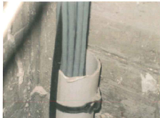
8296_GAINE TECHNIQUE Batiment B2
