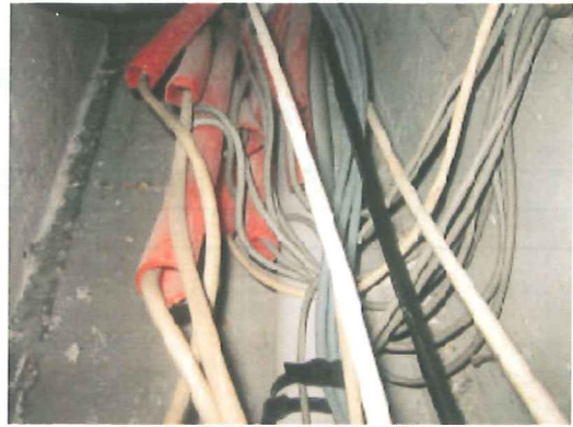
8288_GAINE TECHNIQUE Batiment D
