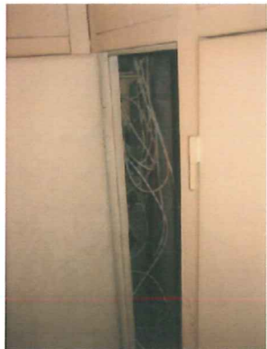
8307_GAINE TECHNIQUE Batiment B1
