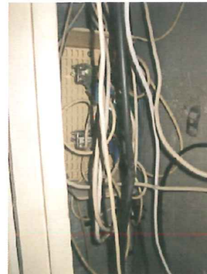
8286_GAINE TECHNIQUE Batiment D
