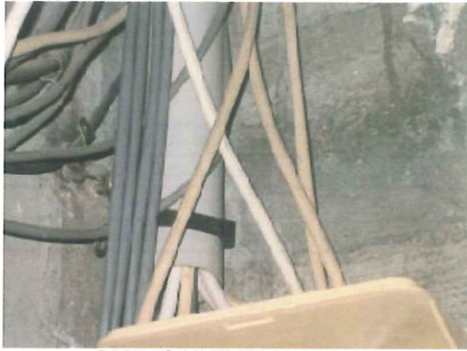
8297_GAINE TECHNIQUE Batiment B2
