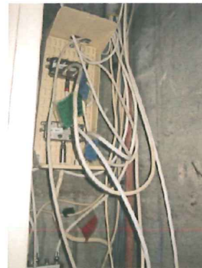
8308_GAINE TECHNIQUE Batiment B1
